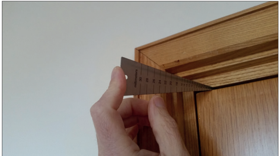
Checking the top edge of a door leaf during a Type 1 inspection. Image courtesy of Golden Thread Fire Delay
