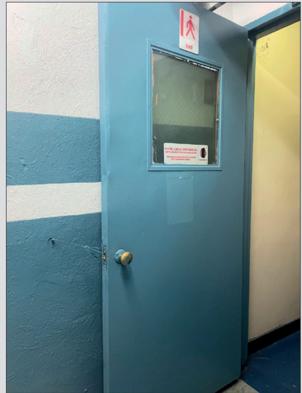
A familiar sight of an old doorset beyond its intended life with no potential for remediation.
