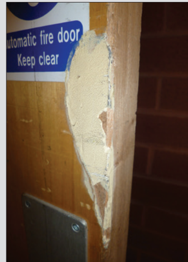
An extreme example of a door leaf in need of replacement.
