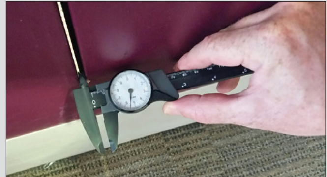
Checking a double door meeting gap with dial calipers during a Type 2 inspection.
