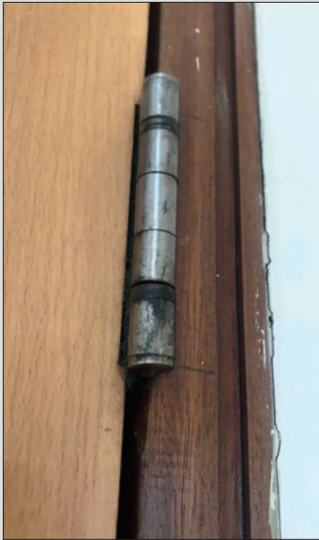
A hinge which has sediment buildup and grime due to lack of maintenance.
